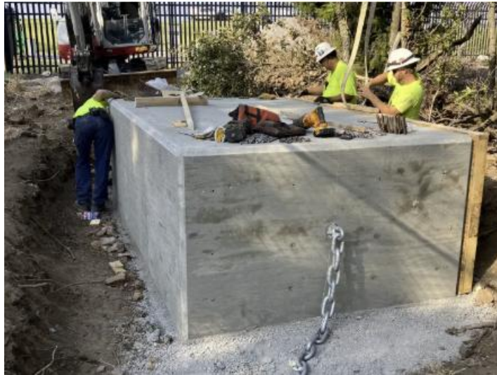
Figure 4. Example on anchor block under construction. Backfill would be expected to minimize the aesthetic distraction of the concrete block.
